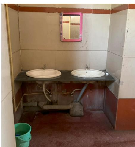
A general area of a female public toilet with two wash basins and one mirror situated at a very elevated height. The picture also shows a bucket filled with water, supposedly to be used in case the water runs out.
