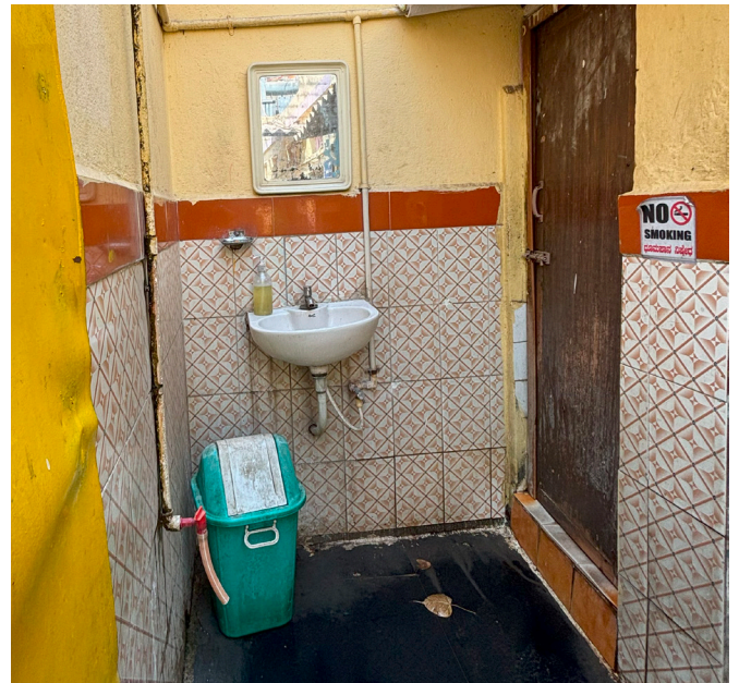
A locked and non-functional stall in one of the public toilets, situated on an elevated platform. The general area also has big-sized dustbin a mirror at an elevated level.
