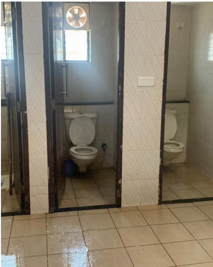
A public toilet in Cubbon park consisting both sit down and western styles of toilet, with a slippery floor and a non functional light bulb.
