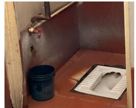
A sit-down toilet with a recycled paint bucket of blue color, used for manually flushing the toilet after each use.
